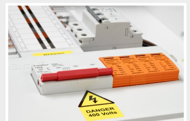
SPD mounted beside main switch
